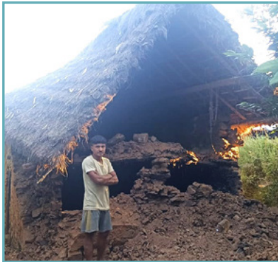
Image: Rukum Earthquake Damaged home
